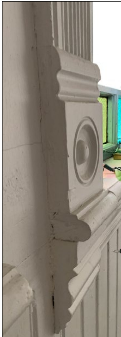
Photo 17 of 18: Additional 1892 moulding detail showing fluted casing, rosettes, bullnosed window stool, corner blocks, chair rail and wainscoting.
