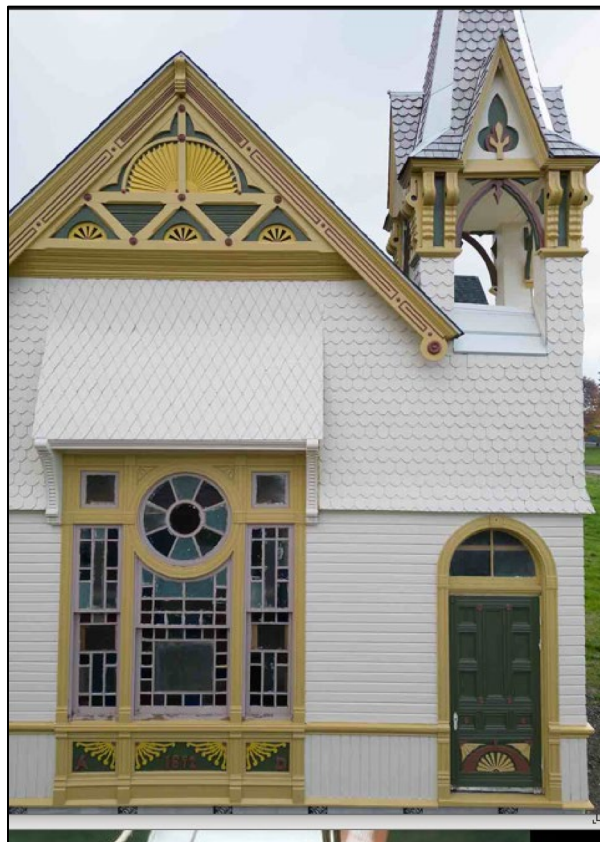
Photo 8 of 18: North façade ganged window unit, gable, bell tower and entry door, camera facing south
