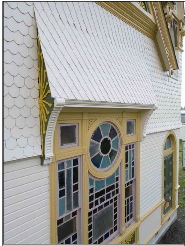
Photo 7 of 18: North façade ganged window unit, window hood, rose window, shingle patterns, camera facing southwest
